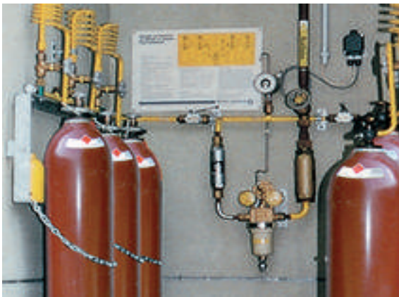
Switchable cylinder bundle station
