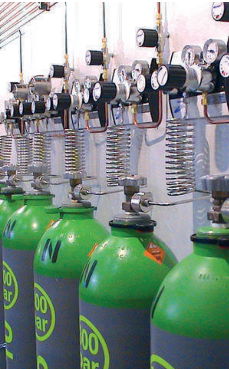
Central gas supply - gases on tap
