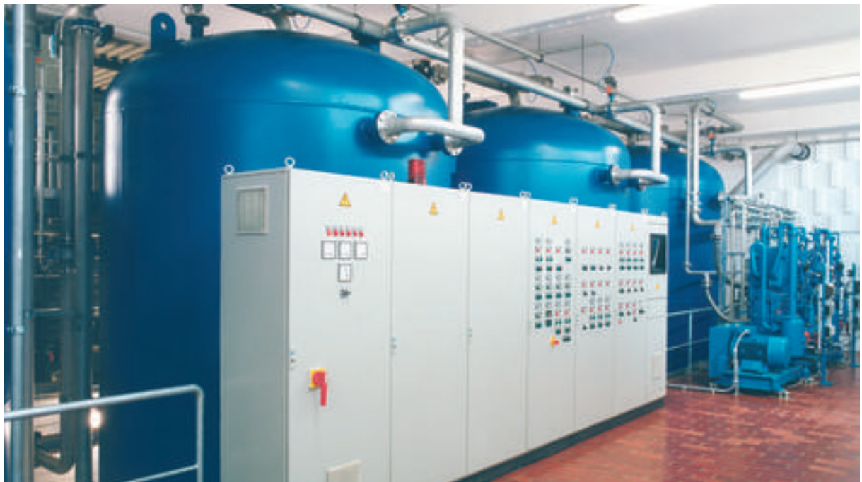
Figure 8: Carix® plant with a capacity of 3000 m 3 /day
