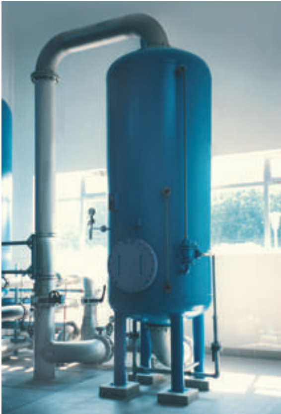
Figure 9: Oxygen injection with an oxygenator for iron and manganese oxidation
