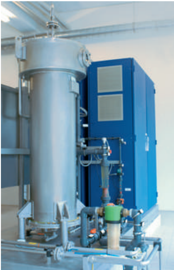
Figure 10: Modern ozone generators like this 3 kg/h installation use pure oxygen as feed
