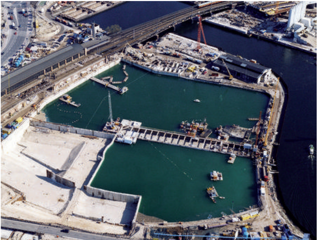
Fig. 4: CO 2 operated construction site neutralization at Berlin's Main Station, former Lehrter Station.
