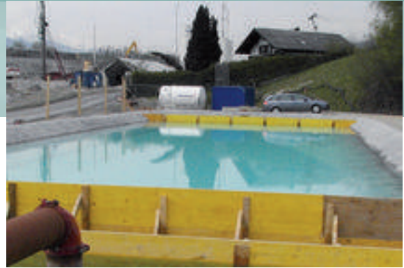
CO 2 storage reservoir of a construction site neutralisation plant
